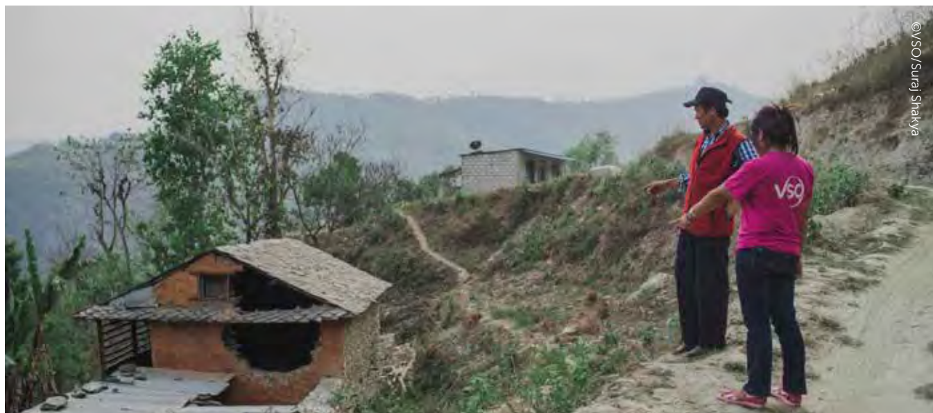
Assessing the damage following the 2015 Nepal earthquake
